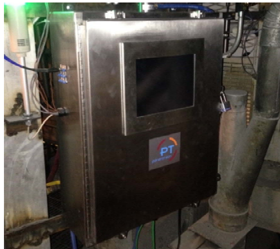
Figure 8. Control box for in-situ probes installed at Libbey, Toledo, OH.
